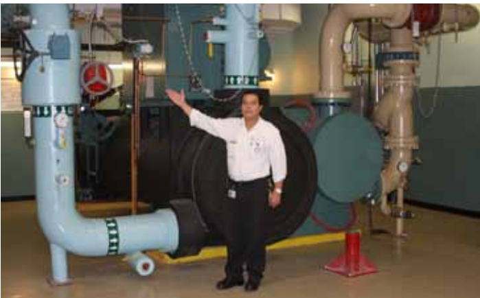
Tony Sousa, Chief Engineer with the 1200 tons dual drive refrigerant unit
