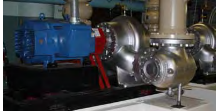
Condenser Water Pump
